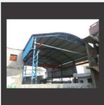
Doom type Fabrication Structure
