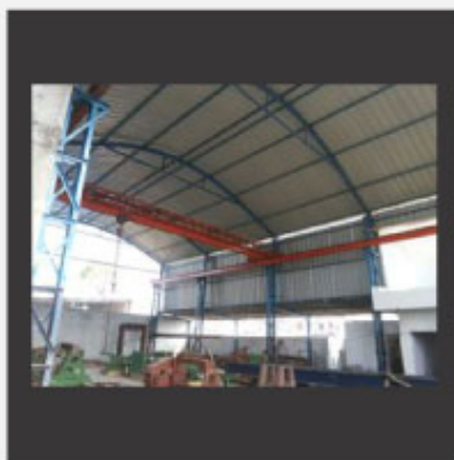
Doom type Fabrication Structure
